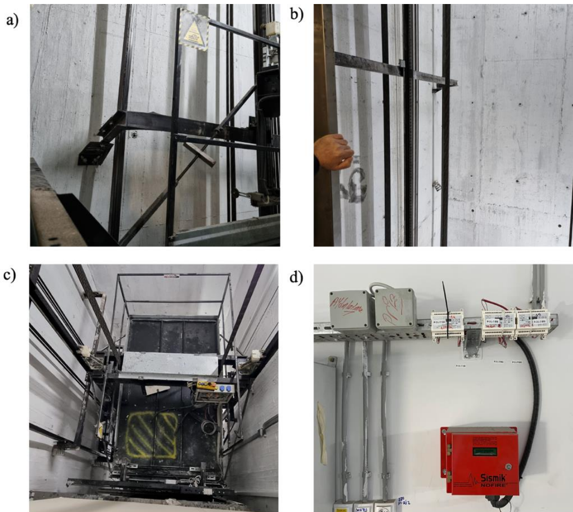
Figure 3 Damage and seismic safety observations in hospital lifts after the 2023 Kahramanmaraş earthquakes: (a) guide rail bracket deformation, (b) damaged bracket region, (c) car, and (d) seismic sensor installed in the lift system
