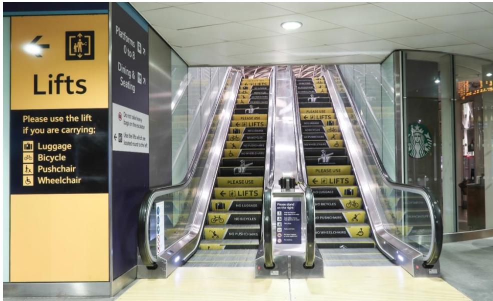
Figure 6 Escalators with low-coefficient step riser panels (which can be advertising or safety signs)
