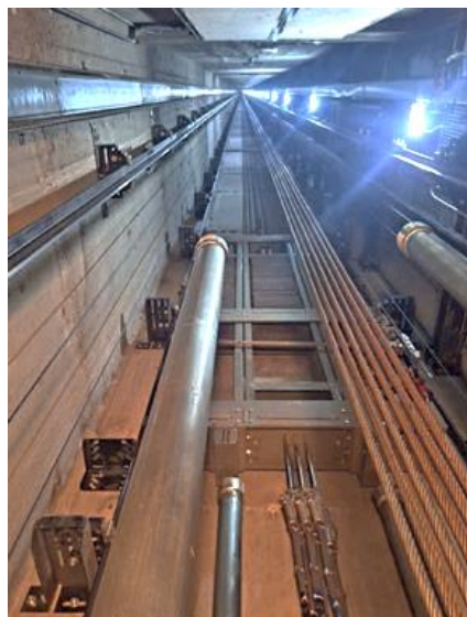
Figure 2: Lift Shaft in Hong Kong (Travel Height > 300 m)
