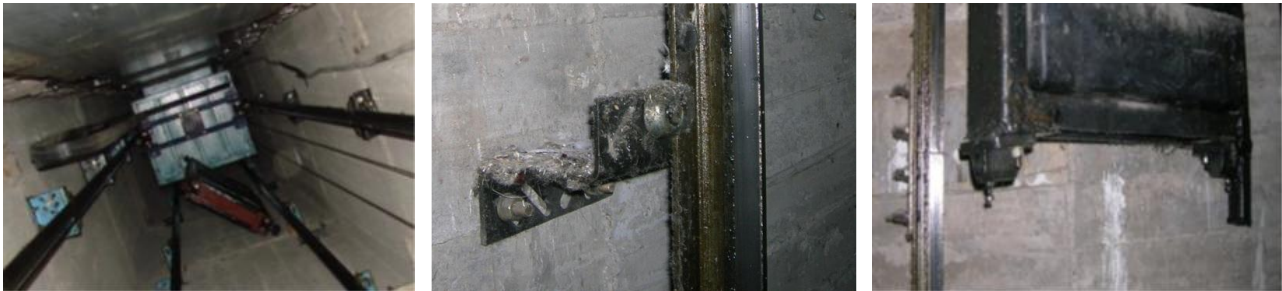
Figure 3 Lift damage of the Van Earthquake [6]
