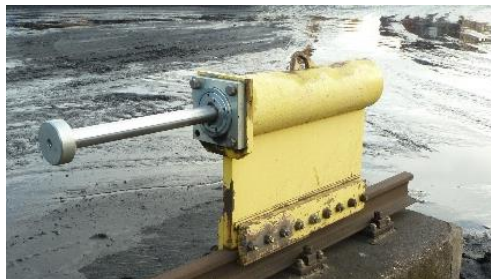
Figure 1 Crane track limit buffer
