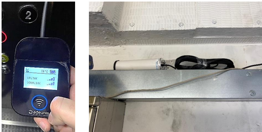
Figures 6a&b ALLIoT field test device and antenna extension
