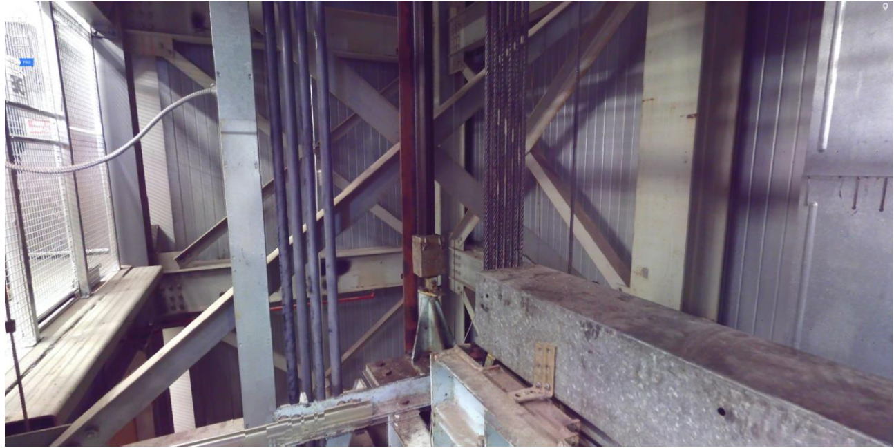
Figure 8. Processed point cloud of a lift shaft taken from the top of the car. [9]
