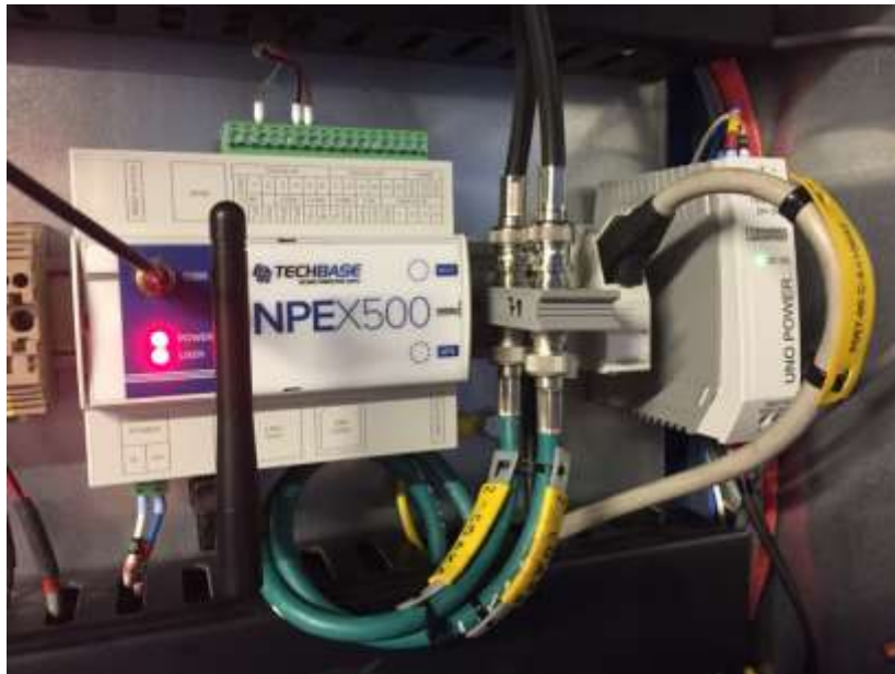
Figure 5 NPE X500 installed on Lift 2
