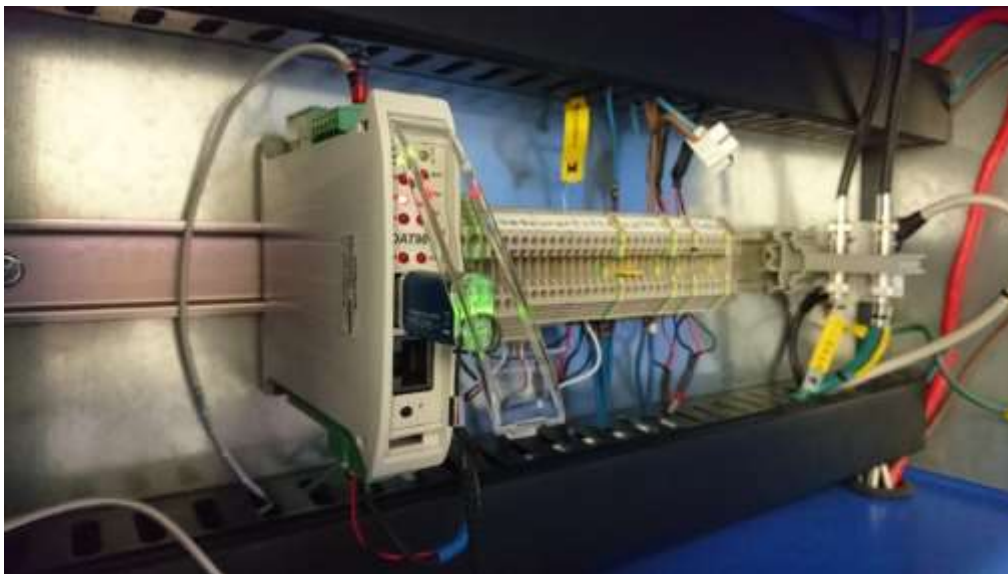
Figure 1 Offline data logger on Covent Garden Lift 1
