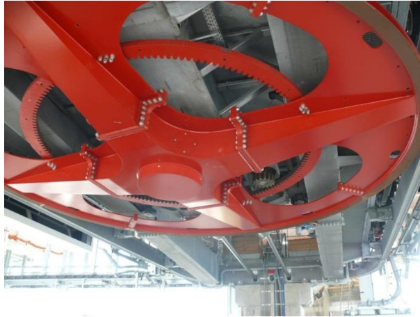
Photograph (5) The main “bull wheel”* and tensioning system in the south station.
