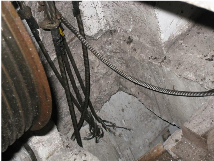
Photograph 2: Failed hoist ropes after dynamic loading
